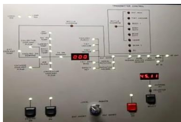
Gambar 2. 4. TCU (Transmitter Control Unit) [sumber: Data Satrad 223 Balikpapan]
